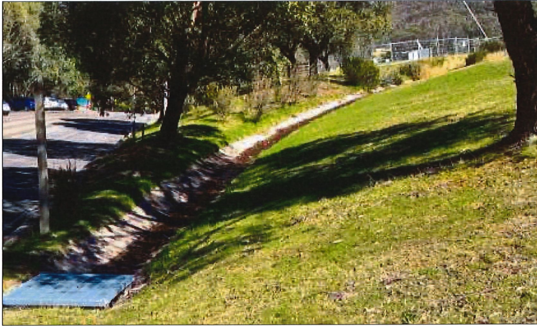
Figure 11: Existing drainage swale – to be diverted with new proposal (Source: Department inspection)
